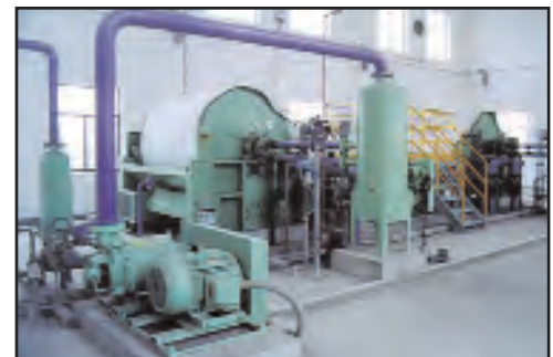
Drum Filter Vacuum System
