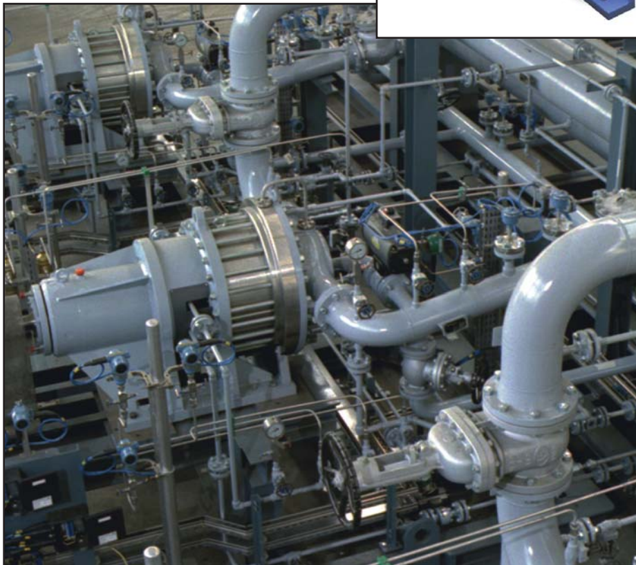
NAB1500 Compressor Package
